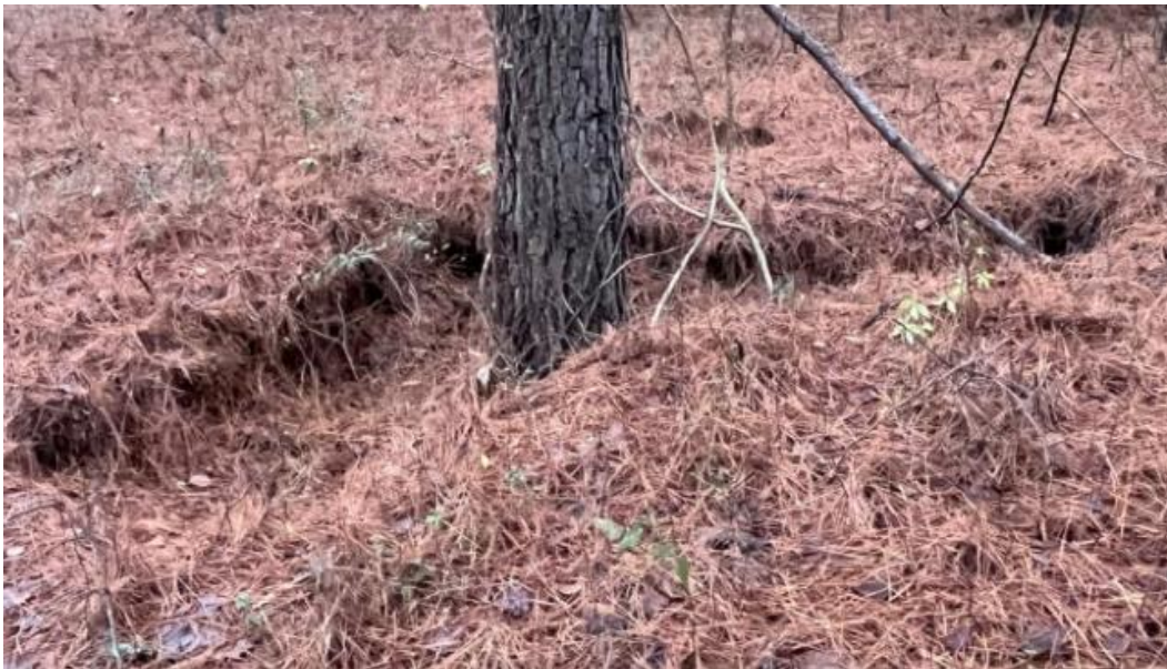
Damaged pipe Sta 6018+25 US end
