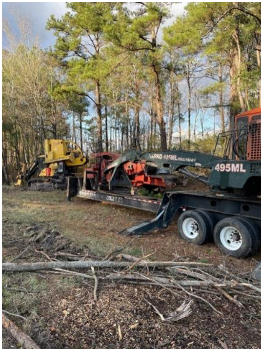
Culvert 1 (Sta 3145+00) DS blocked by equipment
