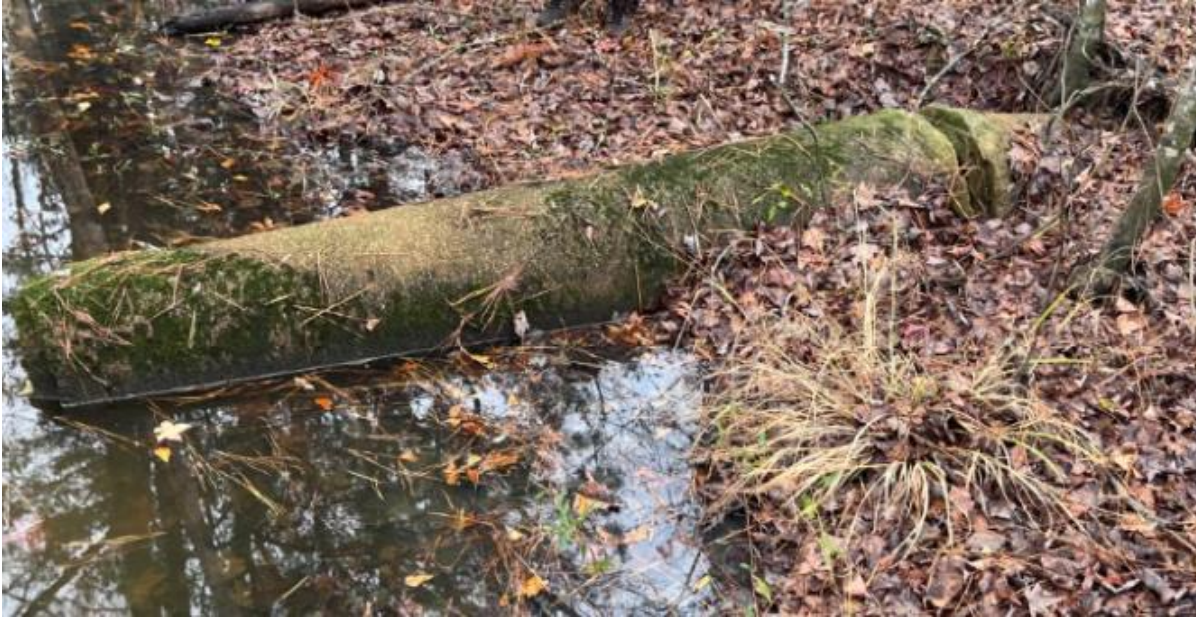
Damaged pipe Sta 6018+25 DS end
