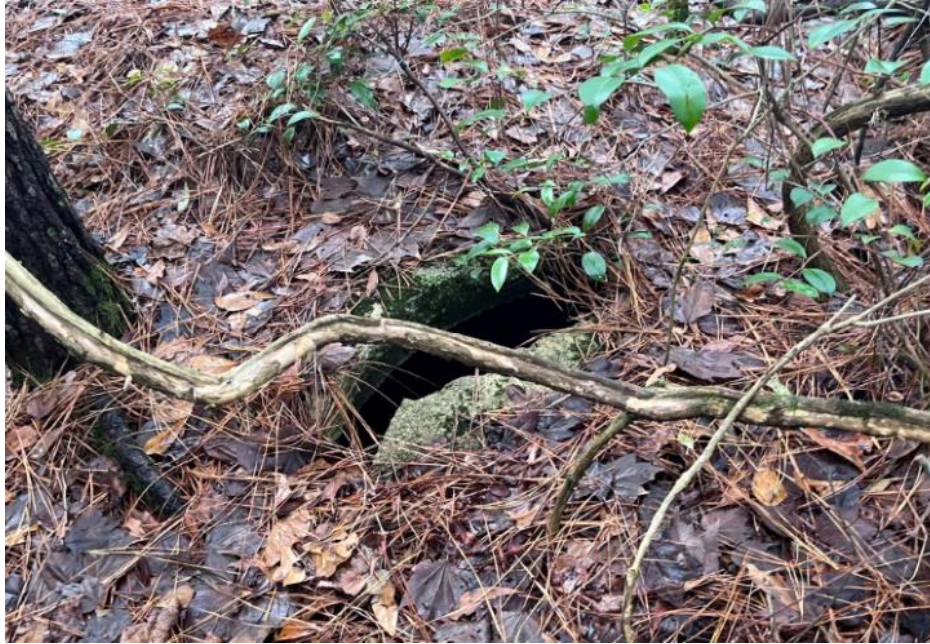
Damaged pipe Sta 5958+00 (I-95 NBL)
