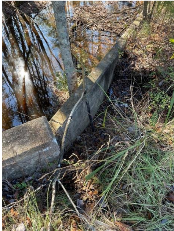
Culvert 3 (Sta 3214+28) US erosion behind wingwalls
