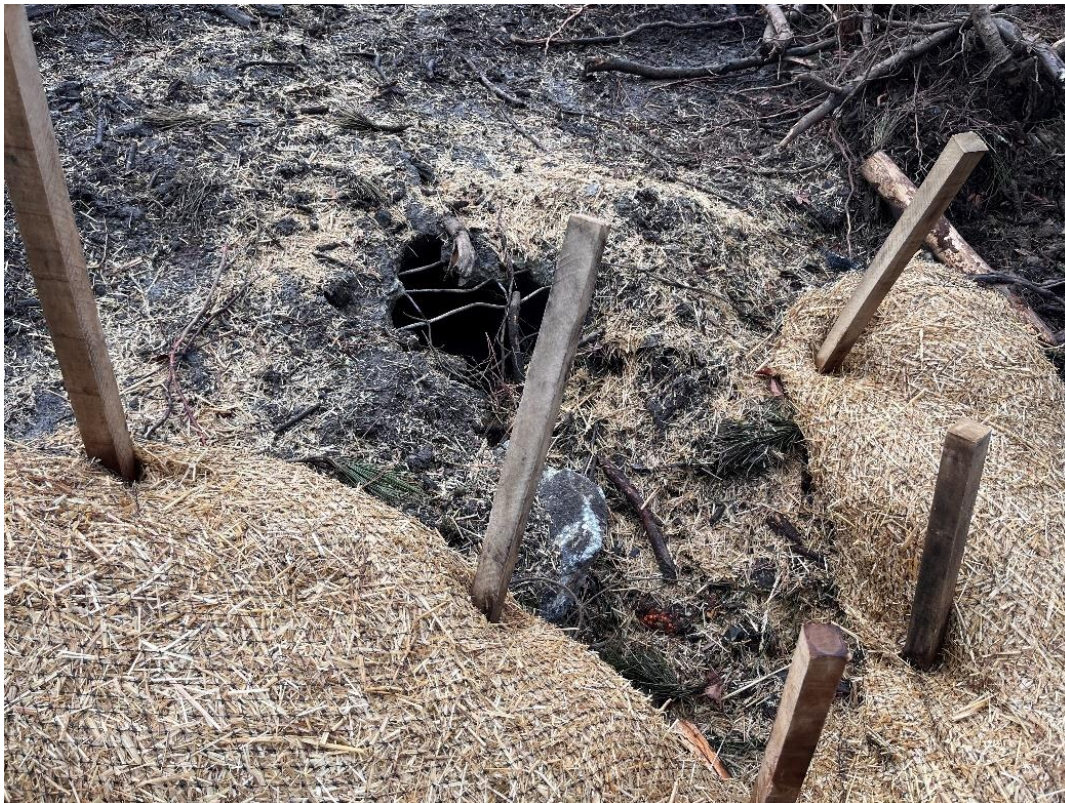
Damaged pipe Sta 3252+00
