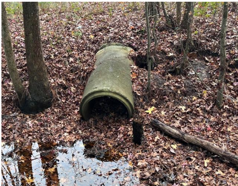
Damaged pipe Sta 5958+00 (I-95 SBL)
